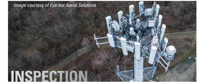
Reality modeling for inspections provides key information, saves time, reduces costs, and minimizes the risk of injuries.
